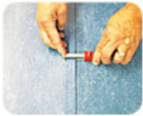
The use of scribing tools can help an installer in the process of fitting and seaming heavy duty materials such as the natural linoleum floor shown here. A wall scribe or recess scribe makes a mark in the surface of the flooring material that becomes a guide for an accurate fit at a wall or a seam. (Photo courtesy of Tarkett)
