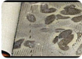
Soft setting adhesives can displace from heavy loads, causing indentations to appear in the surface of the floor covering.
