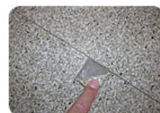
The gaps in this recycled rubber tile installation were caused by too long an adhesive open time, as shown by the visible trowel notches on the substrate that had hardened before the floor was rolled.
