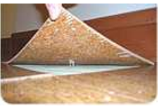
This cork tile installation was curling because the trowel applied adhesive was left open for too long, as shown by the lack of adhesive transfer to the back of the tile.
