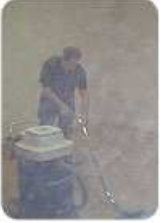
Creating dusty conditions on a job site creates hazards for the installer, the other trades and the occupants of the building.
