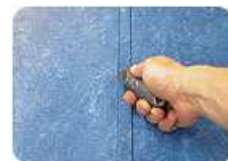
Cutting seams in natural linoleum requires different techniques such as holding the knife at an angle instead of perpendicular to the floor. Photo courtesy of Tarkett.
