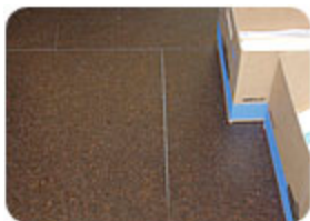
This floor was unprotected after installation, so tiles shifted, the surface got scratched and when they sanded the drywall the scratches
