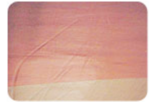
Too much adhesive was used on this sheet vinyl installation so it never quite set up, and a day later when furniture got rolled in, it left marks behind because of the soft and still wet adhesive. Photo courtesy of Peter Austin.
