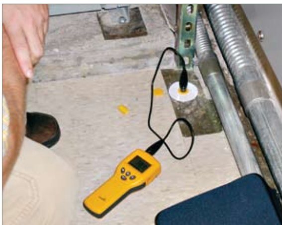
Because this test measures moisture inside the slab, it can predict future moisture movement from inside the slab to the surface.
