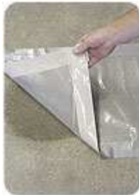
This photo shows a positive result of a plastic sheet moisture test, but doesn't tell how much moisture is present, so more testing I necessary. It's also important to note that a dry result of this test may not necessarily mean the slab is dry. (Photo Courtesy of CTL Group)
