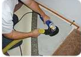
Proper preparation, including grinding the slab, is often overlooked when conducting Calcium Chloride Moisture tests. If this step is not done, the results will not be accurate. (Photo Courtesy of George Donnelly)
