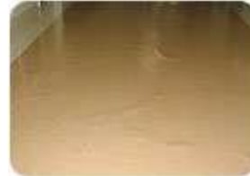
When the old Vinyl Asbestos Tile in this hospital corridor was replaced with Sheet Vinyl, it was assumed that an older building would not have a moisture problem so no testing was done. This shows that ALL slabs need to be tested!
