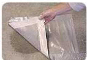
Methods like the plastic sheet test are not acceptable for deciding if a concrete slab is ready.
