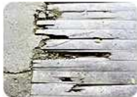
This photo shows why it is crucial to visit the job site before quoting floor preparation. Photo courtesy of Dave Stafford.
