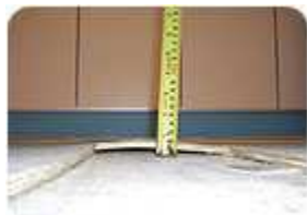
Failure to sufficiently nail the plywood underlayment on this job caused the floor to buckle, leading to a complete replacement of the vinyl and the plywood.
