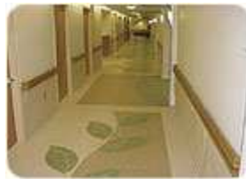
How it should be! Beautiful floor installed over a well-prepared substrate. Photo courtesy of Kevin Mays.
