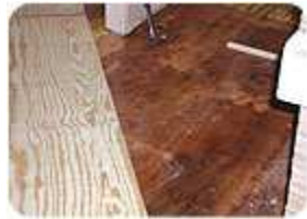
A/C Plywood being installed over an unsuitable plywood subfloor. Photo courtesy of Mickey Moore - FCI October 2004.
