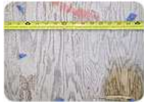
The blue tape shows the nailing pattern on this plywood underlayment - nails are almost one foot apart, so the plywood must be re-nailed every 5-6 inches apart and 3-4" on the seams, before the floor can be installed. Photo courtesy of Jon Namba - FCI October 2003.
