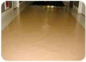
Unfortunately this was a busy corridor in a hospital so cutting open the bubbled sheet vinyl was not practical. An educated guess points to moisture, contamination or other cause of adhesive failure.
