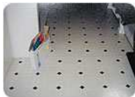
This complaint was easy to diagnose: mismatched sheet vinyl. Photo by Jon Namba.
