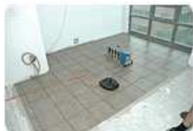
When using a wet set type adhesive, tile must be set while adhesive is still wet, usually after 10-15 minutes of open time. (Photo courtesy of Expanko)
