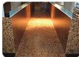
This unique installation of cork on the floors and walls was done using contact adhesive for excellent adhesion on both surfaces.
