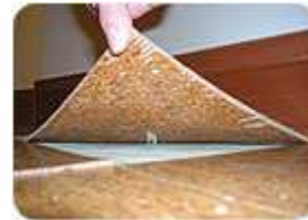
If a wet set adhesive is left open for too long, there will be no adhesive transfer to the back of the tile. Loose, gapped or curling edges are the result.
