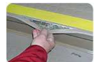
The use of epoxy nose filler can prevent cracking of stair treads.
