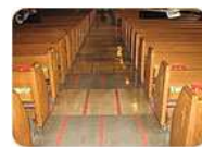
Vinyl Asbestos tile installed in this church in the early 1960's, still in good share today
