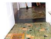
A vintage linoleum floor, circa 1950, was glued to the floor to assure longevity
