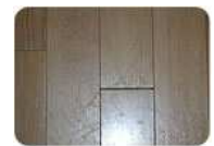
Gapping vinyl plank, vinyl base or vinyl edgings is a condition often caused by installing product that has not been acclimated to job site conditions. Vinyls tend to expand or get stretched when they are handled in very warm conditions, and then they return to their original size when they cool to normal room temperature.
