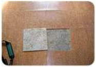
This floor released from the substrate — patching compound and all — because the installer failed to clean the old concrete slab before applying a skim coat. (Photo by Christopher Capobianco)
