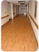
How it should be! This renovation project was done under good site conditions and the substrate was properly prepared so the finished floor was flat and smooth. (Photo by Christopher Capobianco)
