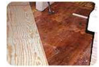
An unsuitable plywood subfloor being covered with new plywood. (Photo courtesy of Mickey Moore - FCI October 2004)
