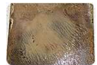
This floor failed because white acrylic adhesive was applied directly over black cutback residue without proper preparation. (Photo by Christopher Capobianco)
