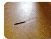
This condition was caused by over-sanding the joints on a properly installed, properly patched plywood underlayment. Sometimes it's possible to overdo it! (Photo courtesy of Mark Violand)
