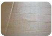
This photo shows a fastener pushing up from the underlayment. Be sure your fasteners are set flush before you install the floor. (Photo courtesy of Bill Baxley - FCI May 2005)
