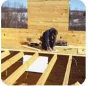
A plywood subfloor is installed directly over the floor joists and is part of the structure of the building. (Photo from www.quiltbus.com )
