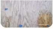
The blue tape shows the nailing pattern on this plywood underlayment - nails are almost one foot apart, so the plywood must be re-nailed every 5-6 inches apart and 3-4" on the seams, before the floor can be installed. (Photo courtesy of Jon Namba - FCI October 2003)
