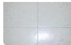
This VCT floor is "running off" so the tiles do not line
