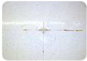
This VCT floor is showing signs of excessive moisture vapor emissions from the concrete and the high alkalinity that comes with it.
