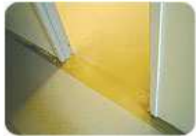
By using a VCT adhesive with long open time, the field tile is installed first and border cuts are done later - often up to 24 hours after spreading the adhesive. (Photo courtesy of Pyramid Floor Covering)
