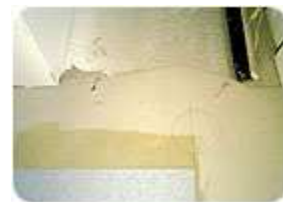
Preparation done right. From top to bottom, this photo shows a rough concrete slab, a self leveling underlayment, clear thin spread adhesive and finished VCT. (Photo courtesy of Pyramid Floor Covering)
