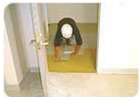
This installer got enough time for floor prep and installation, and the finished floor looked great. (Photo courtesy of Pyramid Floor Covering)
