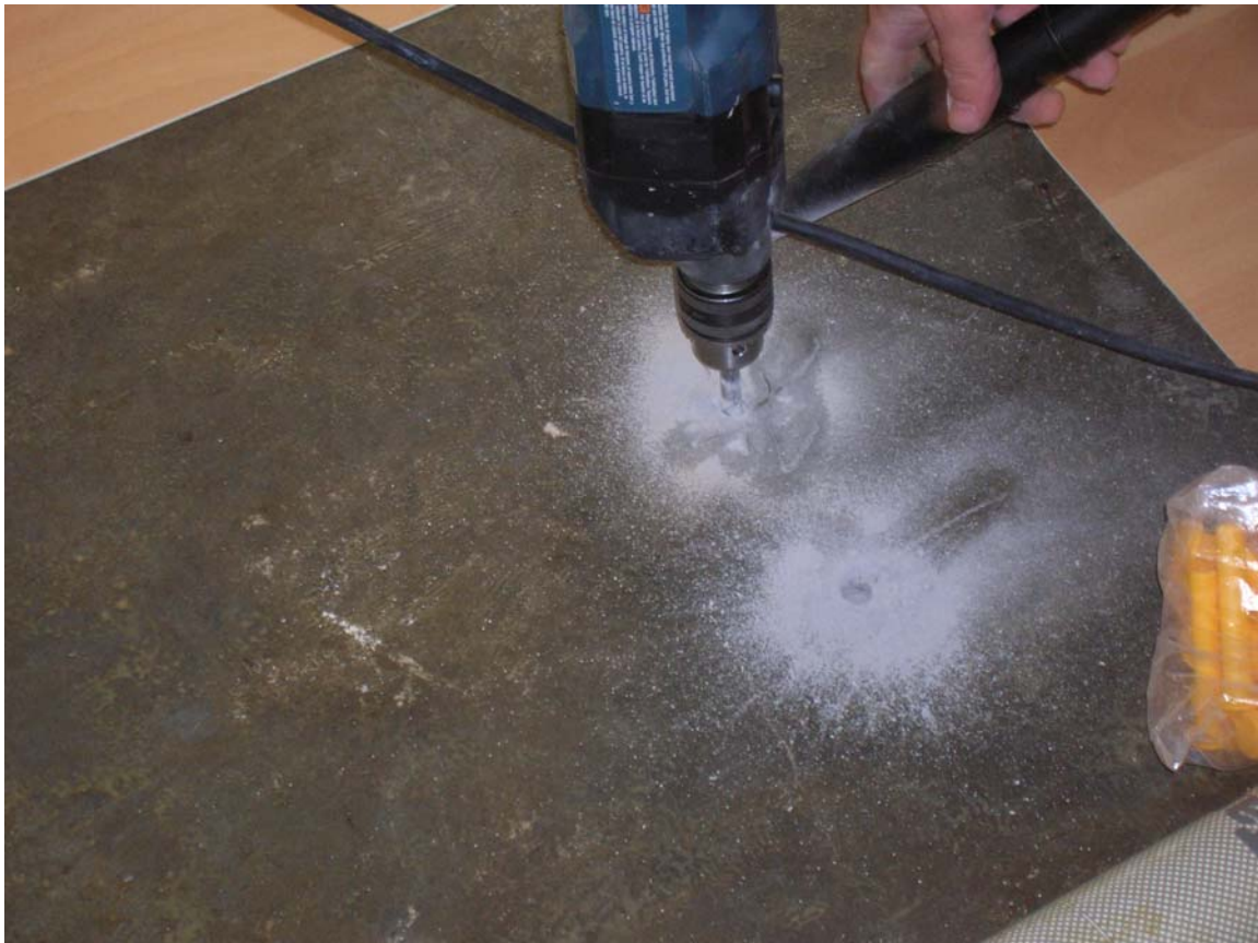
By drilling into the concrete, the ASTM F 2170 method can measure internal moisture levels.
