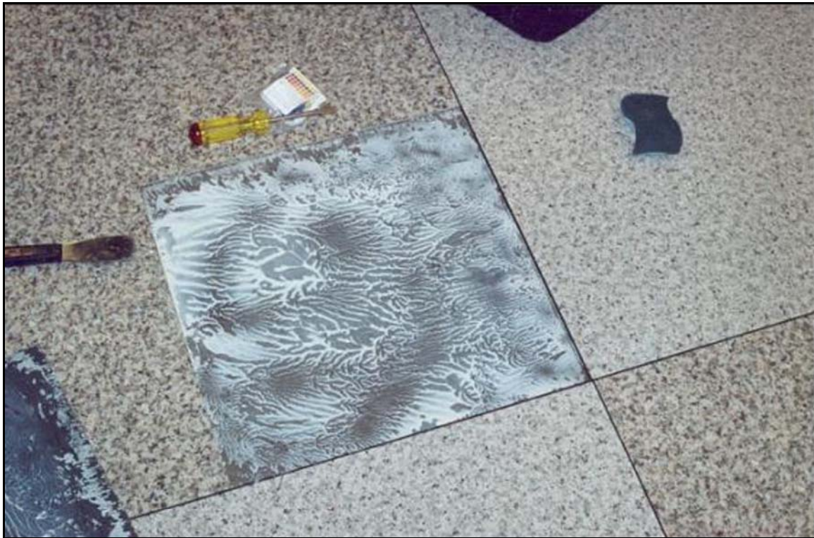
Floor tiles are prone to cracking in severe moisture conditions when the adhesive beneath the tile re-liquefies due to moisture emissions from the concrete.
