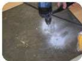
To run the ASTM F 2170 Relative Humidity probe method, first drill a hole to 40 percent of the concrete depth. (Photo by Christopher Capobianco)
