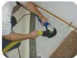
Proper cleaning of the concrete slab before Calcium Chloride Testing is critical for accurate results. (Photo courtesy of George Donnelly)
