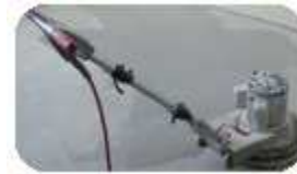
Adequate preparation of concrete includes moisture testing and a light sanding, as shown here.
