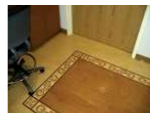
This inlaid border arrived to the job pre-cut, so the installer carefully planned where the inlay would go, had it approved by the owner, and then installed it a section at a time.
