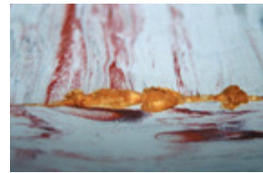
Using the wrong adhesive and a concrete moisture condition caused the ooze on this rubber tile installation. Thanks to Bill Baxley for the photograph.
