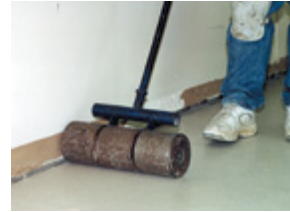
Rolling the floor helps assure adhesive contact and will minimize the chance of air bubbles. Thanks to Ray Thompson for the photograph.
