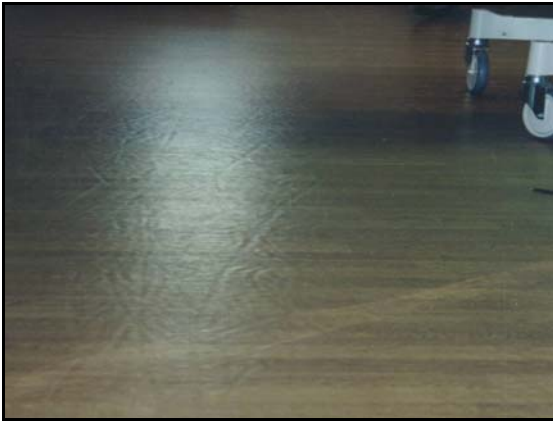
This resilient flooring material is showing wheel marks because the adhesive has softened due to moisture.
