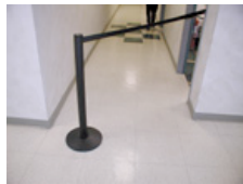
The rubber base on the bottom of this pedestrian control device can leave a stain on a resilient floor when it is left in one place for an extended period.
